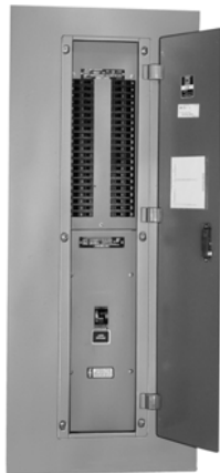
225 A Main Circuit Breaker
